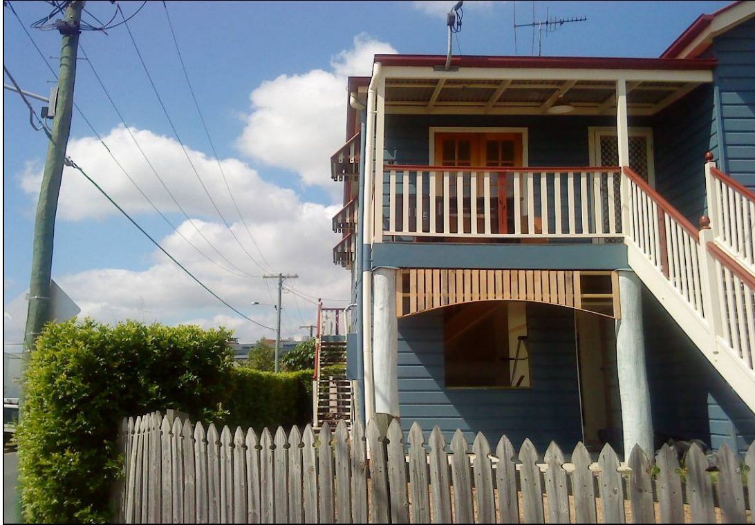
Photo A1: Showing renovations underway at the ground floor level at 6 Albert St, Woolloongabba.
